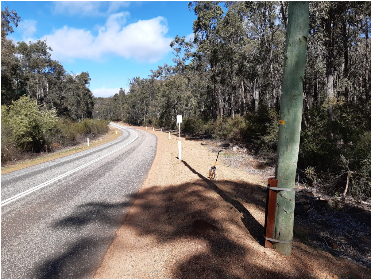
Del Park Road –Tree clearing for Road widening & Overhead power pole relocation
